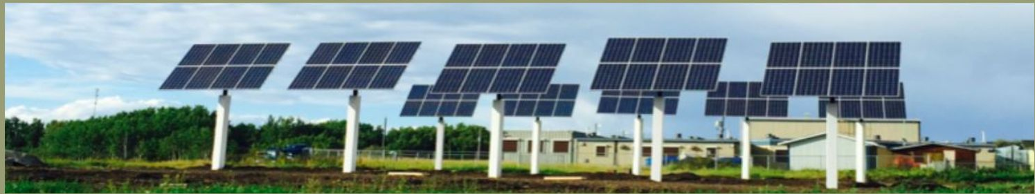
Final Solar Installation – Top of Pole Mount System – 20.8 kW
