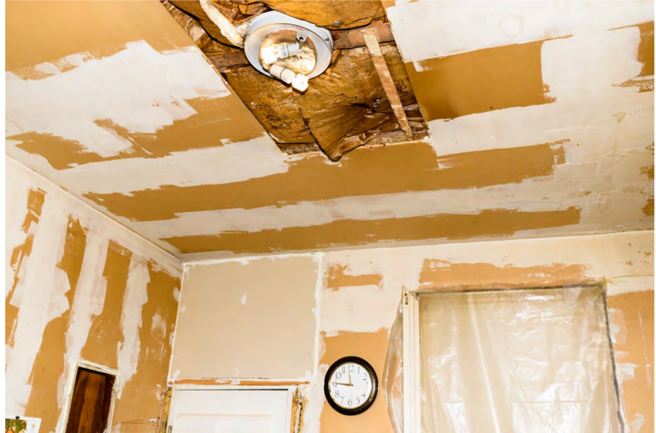
A Kingsessing home after participating in Basic Systems Repair for a roof.
